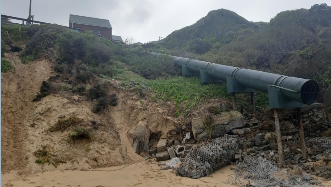
Photograph of exposed infrastructure in Brenton on Sea – Image courtesy of Knysna Municipality.
